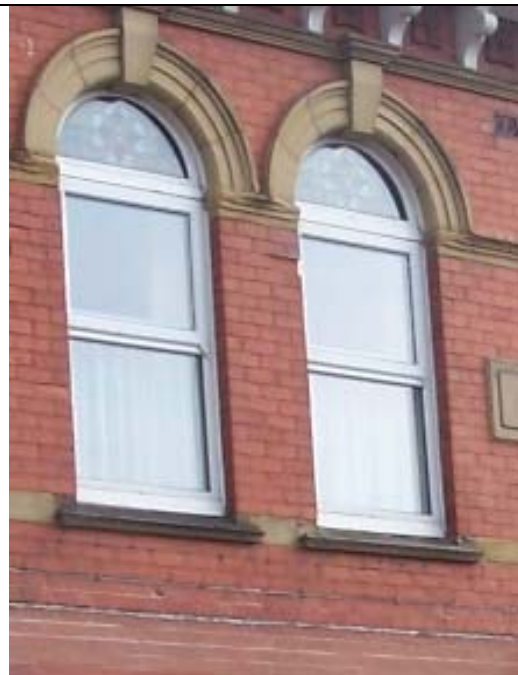
FIGURE 92. EXAMPLE OF INAPPROPRIATE MODERN UPVC WINDOWS
