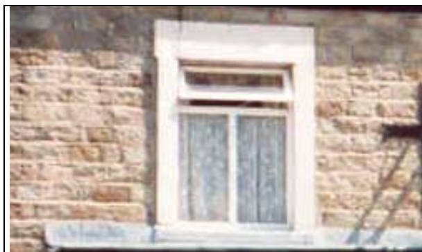
FIGURE 112. INAPPROPRIATE REPLACEMENT WINDOWS
