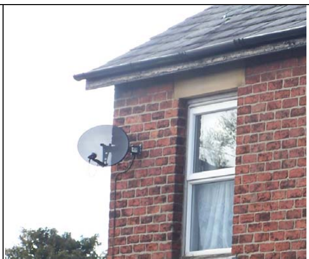
FIGURE 119. INAPPROPRIATELY PLACED SATELLITE DISH
