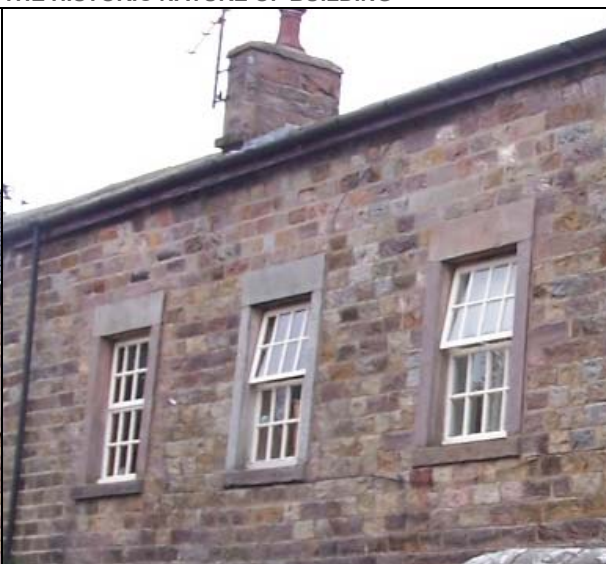
FIGURE 58. INAPPROPRIATE MODERN OUTWARD OPENING MOCK SASH WINDOWS
