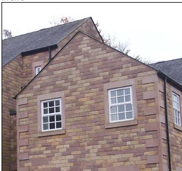
FIGURE 57. INAPPROPRIATE MODERN MOCK SASH AND CASEMENT WINDOWS
