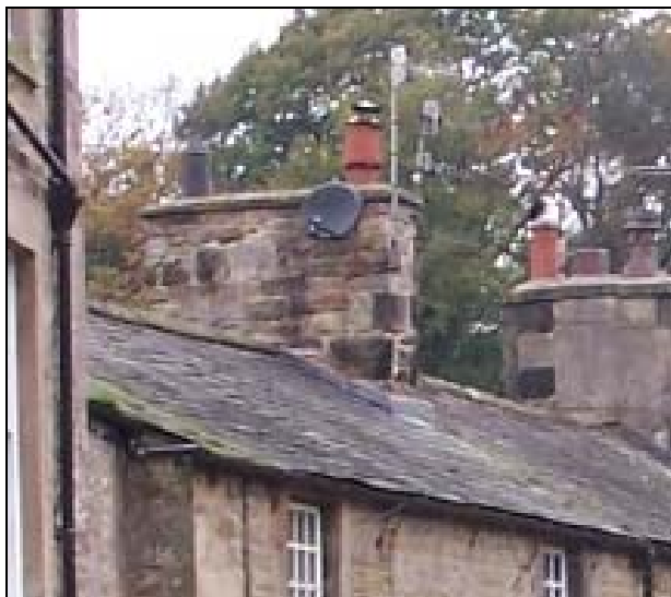
FIGURE 59. INAPPROPRIATELY PLACED SATELLITE DISH
