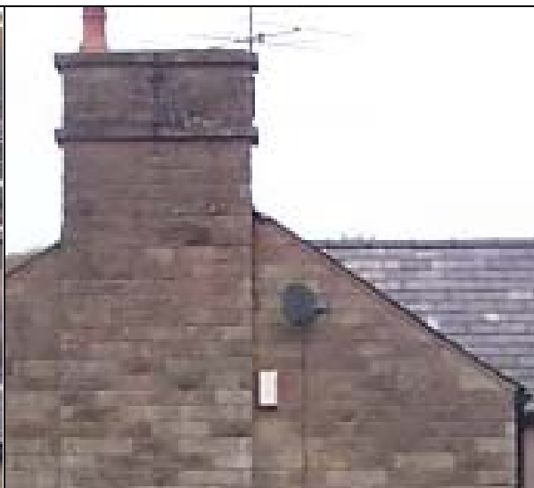
FIGURE 60. INAPPROPRIATELY PLACED SATELLITE DISH
