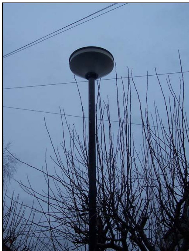
FIGURE 65. MODERN STYLE OF STREET LIGHTING
