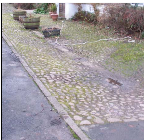
FIGURE 63. REMOVED BOUNDARY WALL CREATING INCONSISTENT OPEN AREAS
