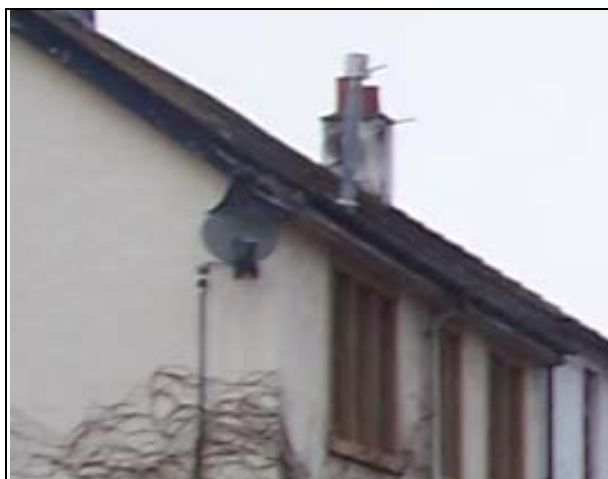
FIGURE 101. INAPPROPRIATELY PLACED SATELLITE DISH
