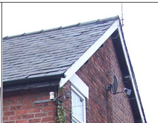
FIGURE 102. INAPPROPRIATELY PLACED SATELLITE DISH
