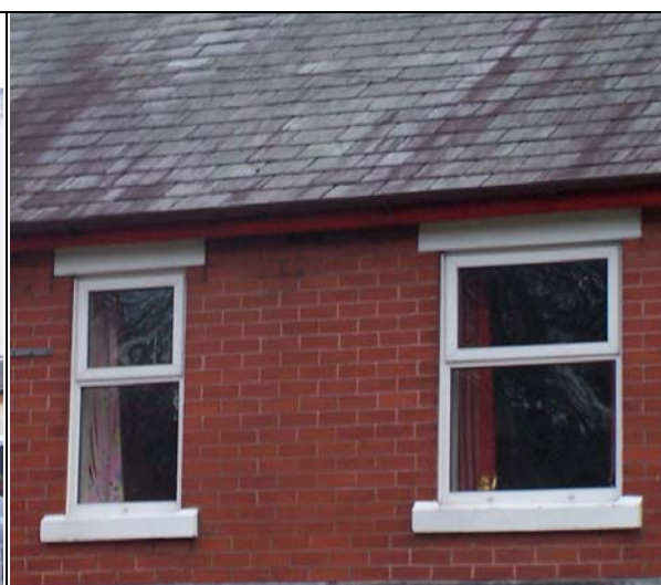
FIGURE 98. INAPPROPRIATE REPLACEMENT UPVC WINDOWS
