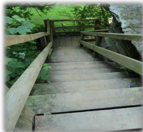
The Wyre Aqueduct wooden steps need attention
