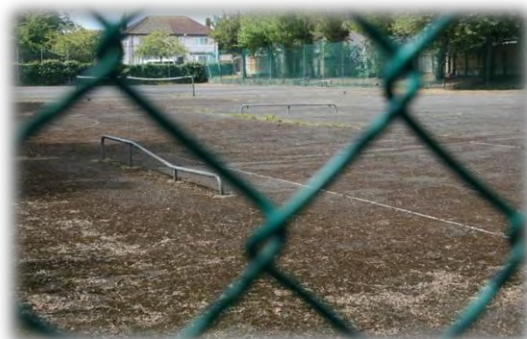
Tennis Courts require upgrading and is being addressed
