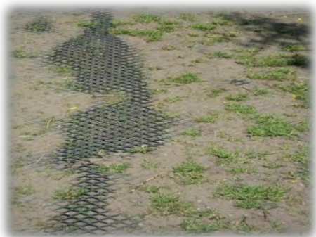
Part of worn out footpath
